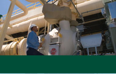
Galena III Geothermal Plant Lyon County, Nev.
